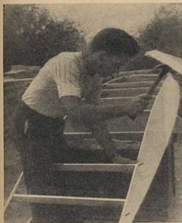
Bottom bracing is put in (above) just after the lower side planks, with nails driven into their ends from the outside
